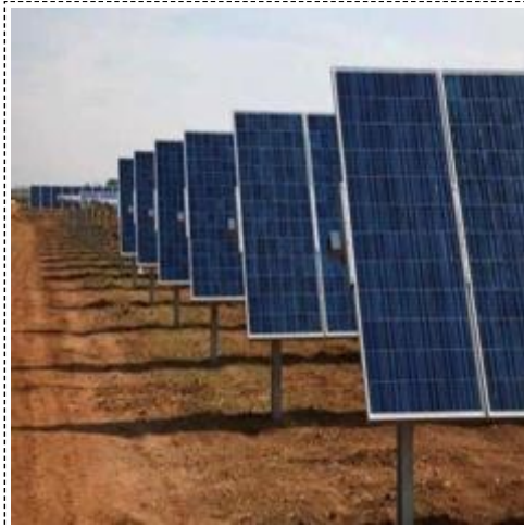
Solar power project studies
