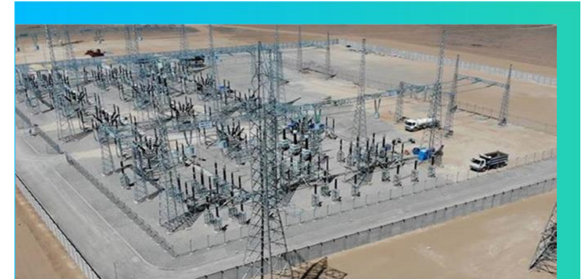
Algarrobal (National) 220 kV sectioning substation Project completed / CEN recognition 08-Jul-2021
