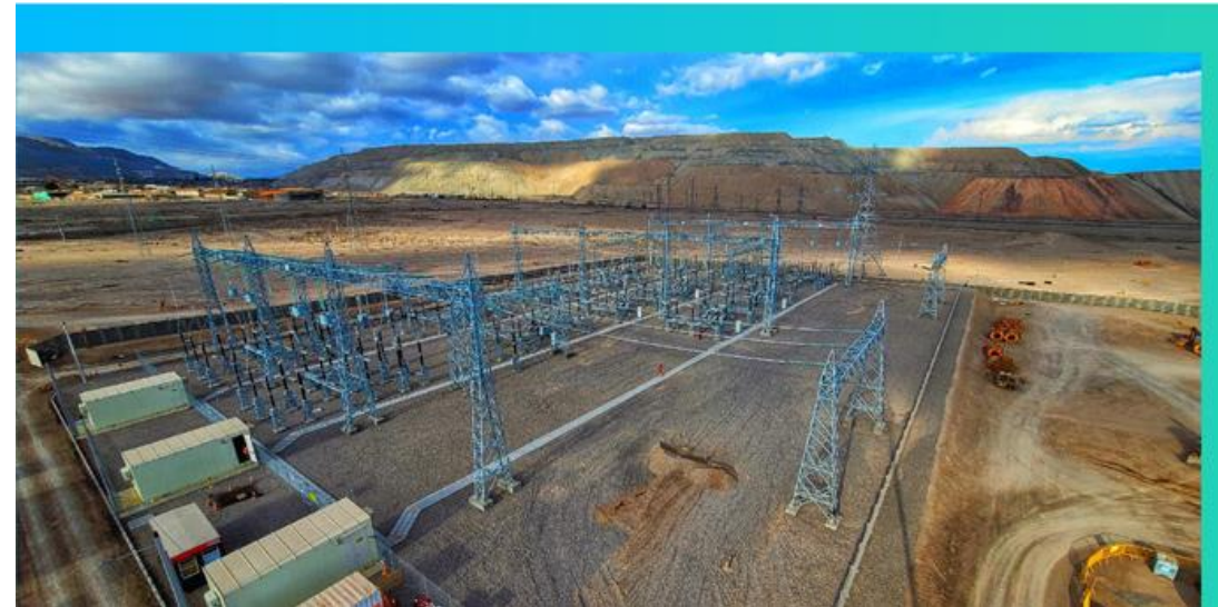
Nueva Chuquicamata (National) Substation + 2 x 220 kV transmission line Project completed / CEN recognition 06-Dec-2021
