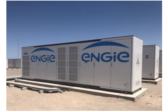
116MW / 660 MWh BESS Tocopilla (storage) US$180 million investment
